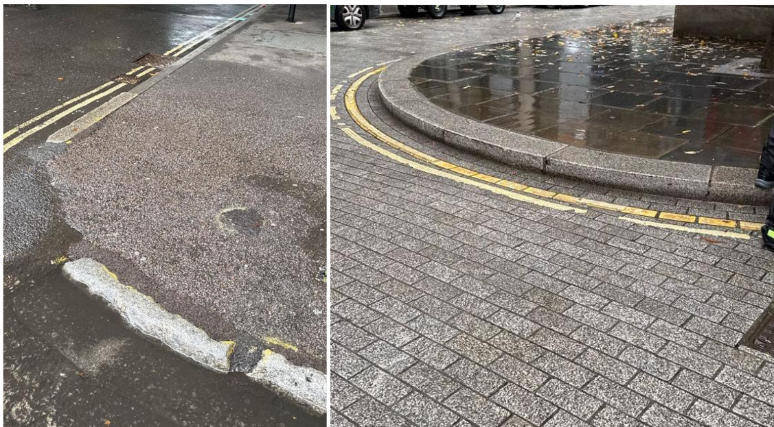
Image 1: Dropped kerb that hasn't been maintained.
