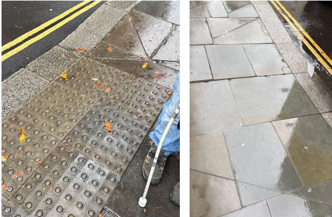
Image 5: Dropped curb with contrasted tactile paving, with no tactile cues on the steep slope on either side. Image 6: Dropped kerb with no tactile paving.
